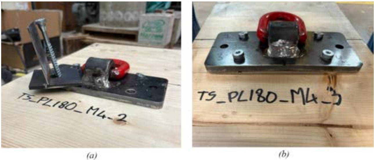
Figure 25. (a) Insertion of the screw at an inclination of 10° using a dedicated jig; (b) Screws in place after installation, inclined at 10° (MECH 4).
